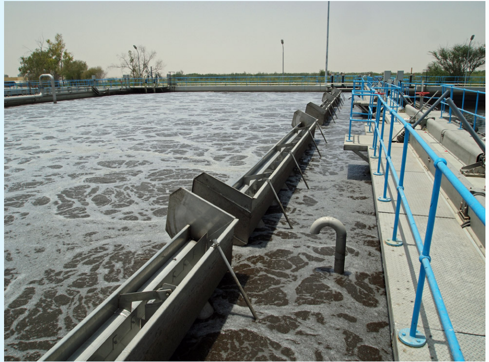
Effluent Decanters - Raised Position in Aeration Phase
