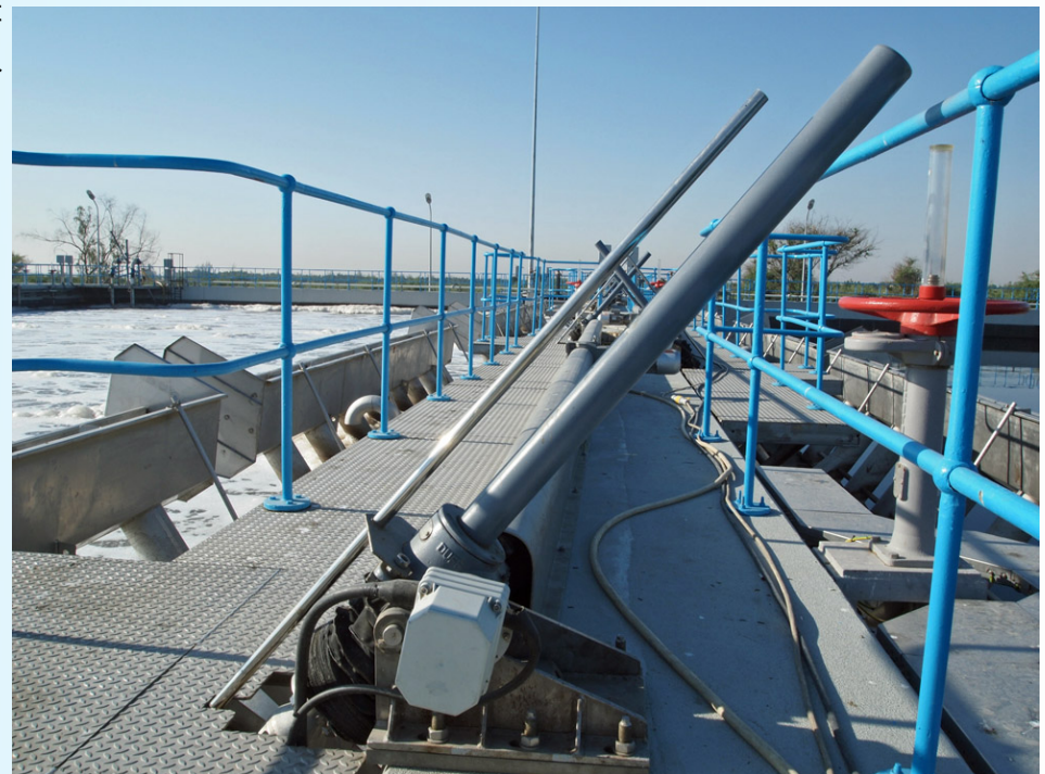
Effluent Decanters - Showing Worm Drive Decanter Lifting Mechanism
